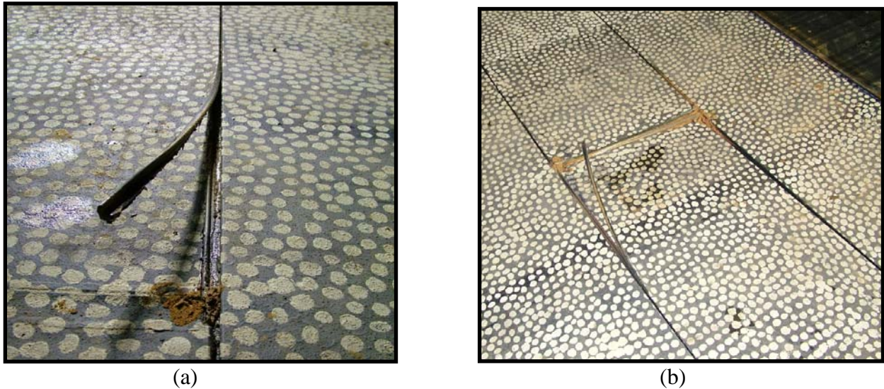
Figure 16: AM-2 failure in the joint rail (a) and relative deflection between panels (b)
