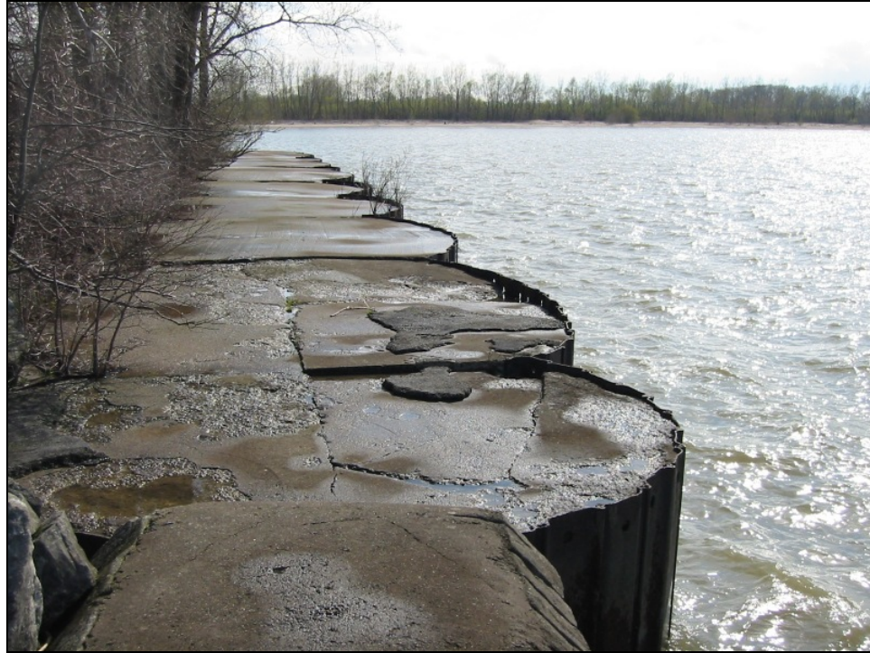
Figure 5. West side of NASA pump facility, 27 April 2005. Barrier beach at nature preserve is in background
