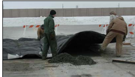
Figure 9. Laying insulation blankets in the wind and holding them down with sand bags.
