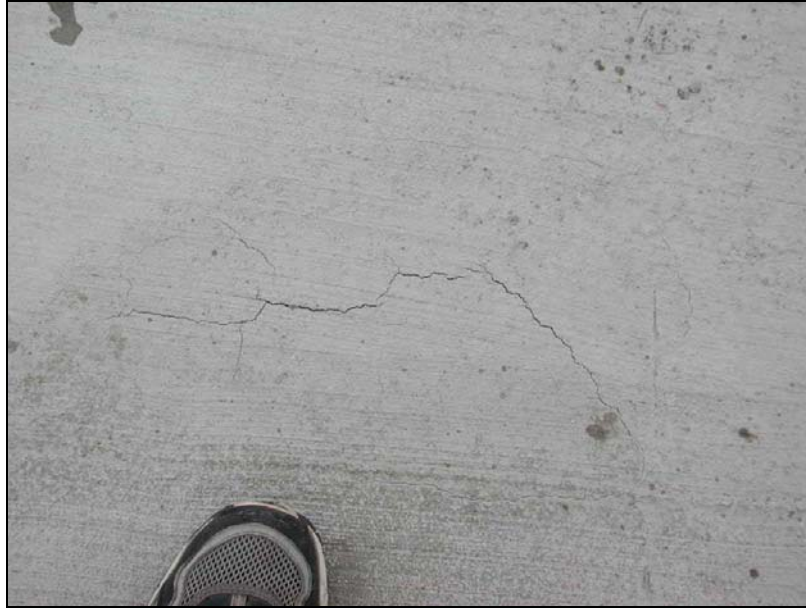
Figure 13. Crack that developed in the concrete approximately 3 hours after the insulation blanket was removed.
