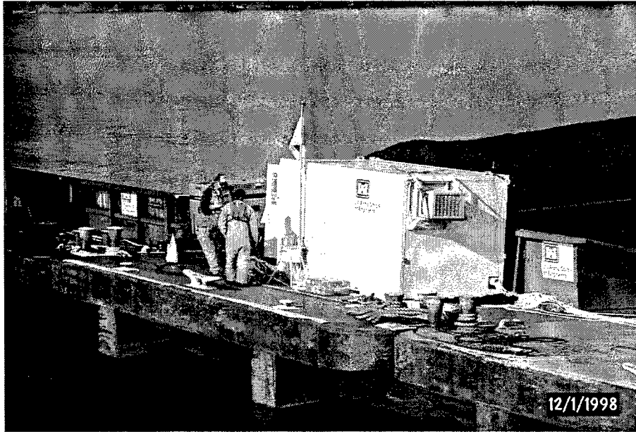
Figure 5.1. Onboard instrumentation enclosure on middle lead barge (Note: barge impact corner is just to the right of the picture)
