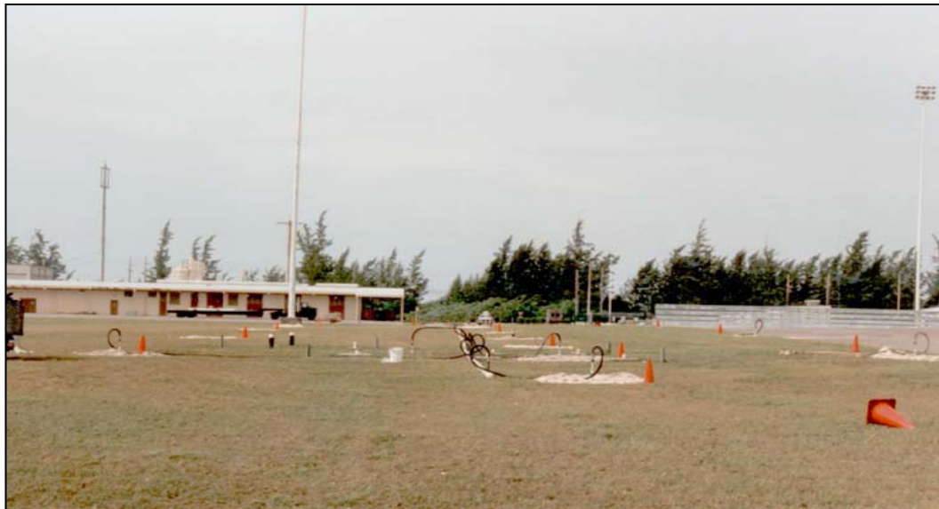
Bioslurper Wells in Grass Area
