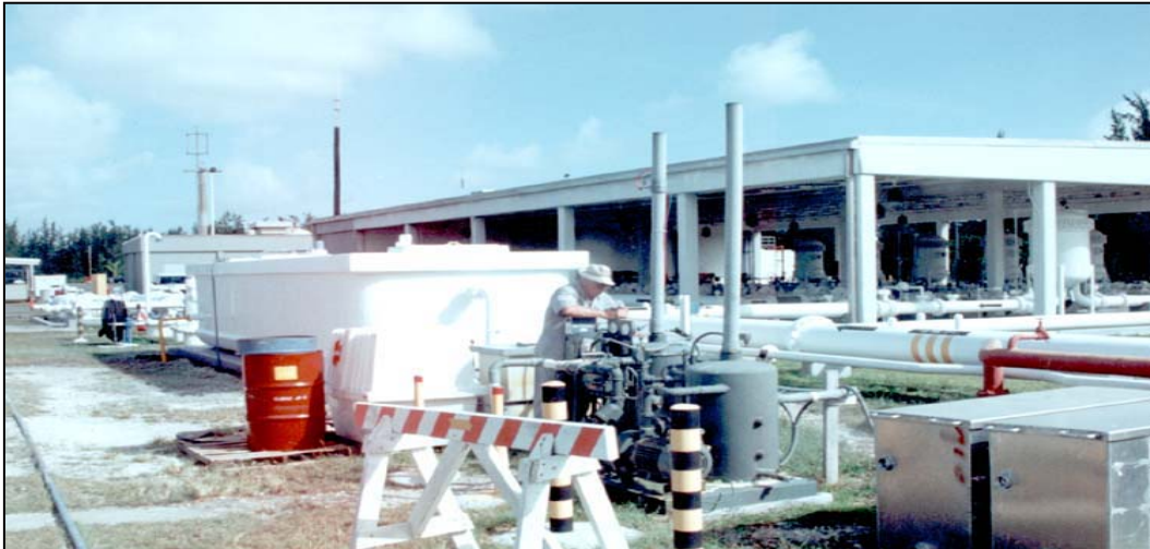
Two Bioslurper Pumps in Fuel Storage Yard
