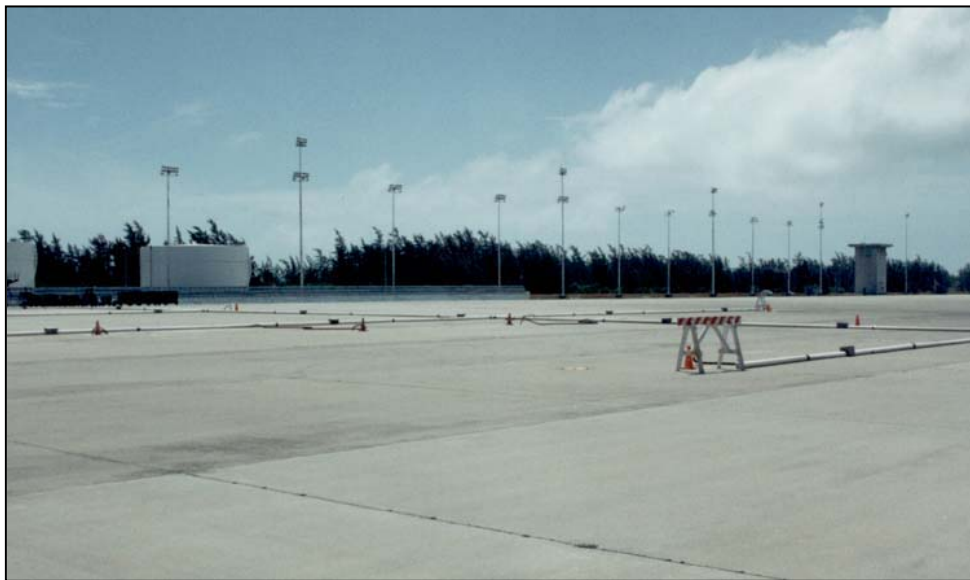
Bioslurper Piping on Ramp
