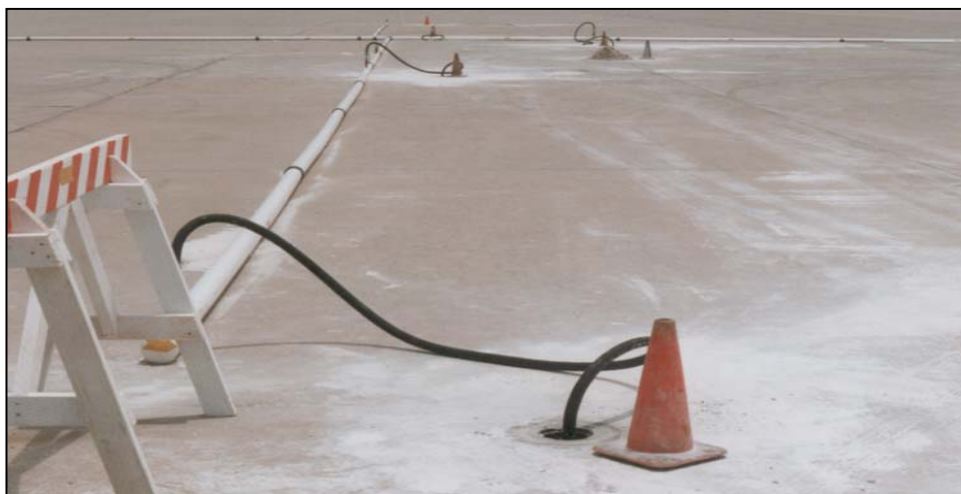
Connection to Bioslurper Well on Ramp
