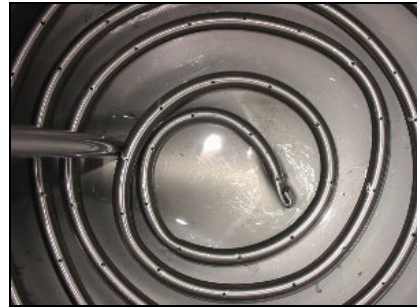
Fig. 3.18 Sparging coil close-up
