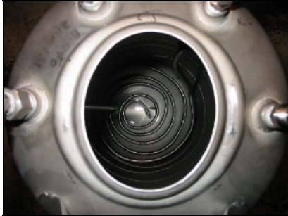
Fig. 3.17 Sparging coil in fuel tank
