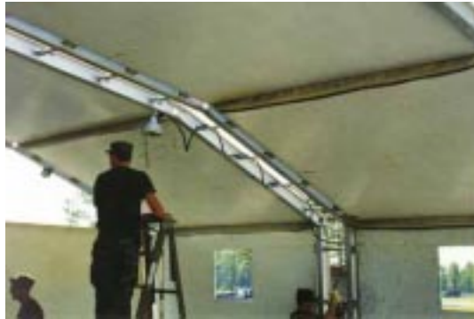
Figure 73. Lighting Fixture Cable Run.
