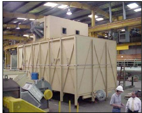
Rear and Side View of Hot Gas Decontamination Chamber
