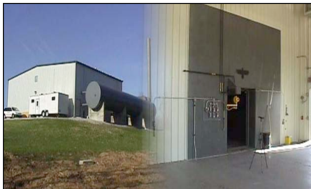
Contained Detonation System
