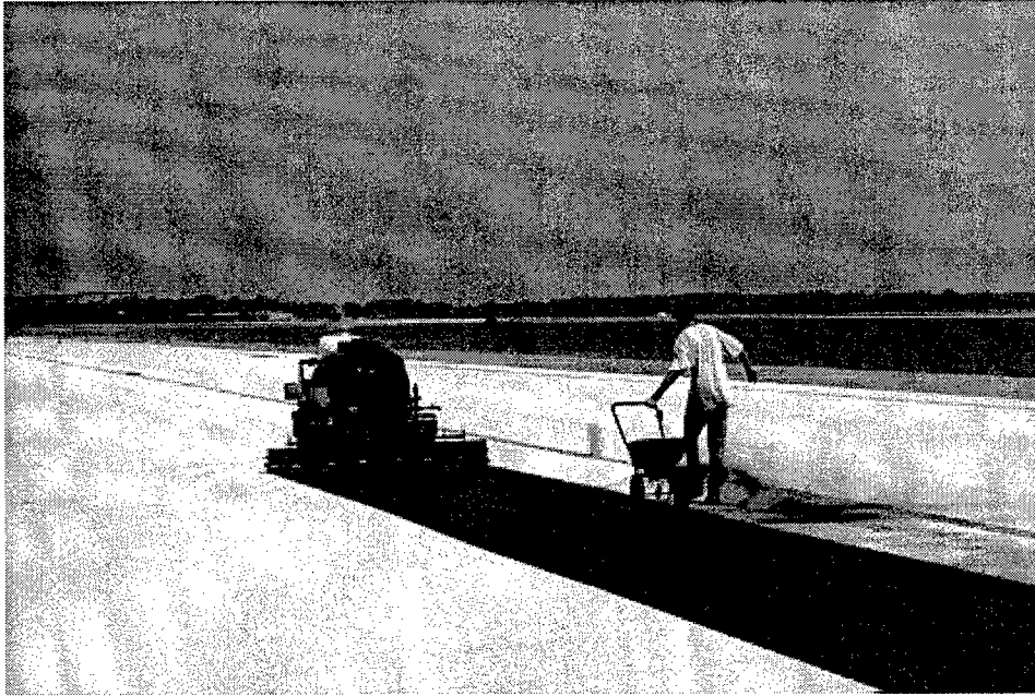
Figure 12. Spray application equipment applying CBRT-SO. Note application of sand to treated surface
