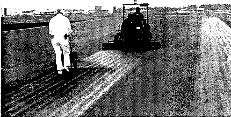
Figure 19. Applying BCR-2000 emulsion, with sand spread by hand-pushed applicator immediately on the treated surface (MacDill AFB)
