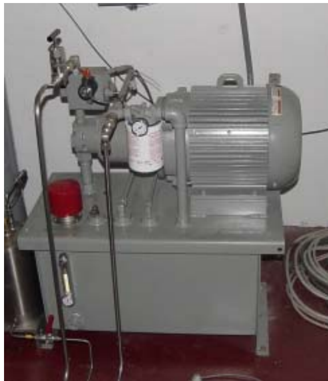
Figure 6. Hydraulic Power Unit
