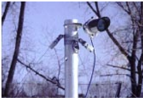
Figure 1. Eltec PIR at IDS field site.
