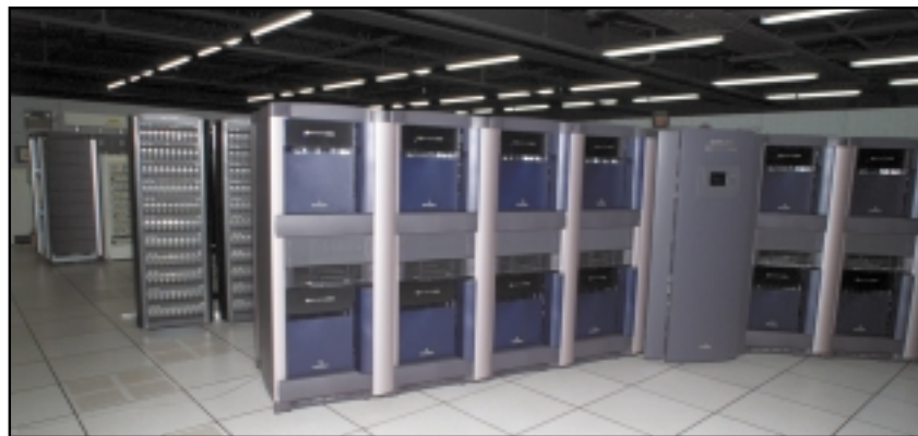
The 128-processor Silicon Graphics Origin2000 system, currently with 128 Mbytes of RAM. The next-generation Origin3000 in the background transitions from beta to experimental use in FY 01. The NRL Center for Computational Science, as a Distributed Center of the DoD High Performance Computing Modernization Program, provides such systems (at no cost) for anyone approved by the Program Office.
