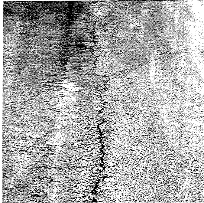
Figure 3.4: Small crack in longitudinal construction joint between lanes of RMP at Malmstrom AFB
