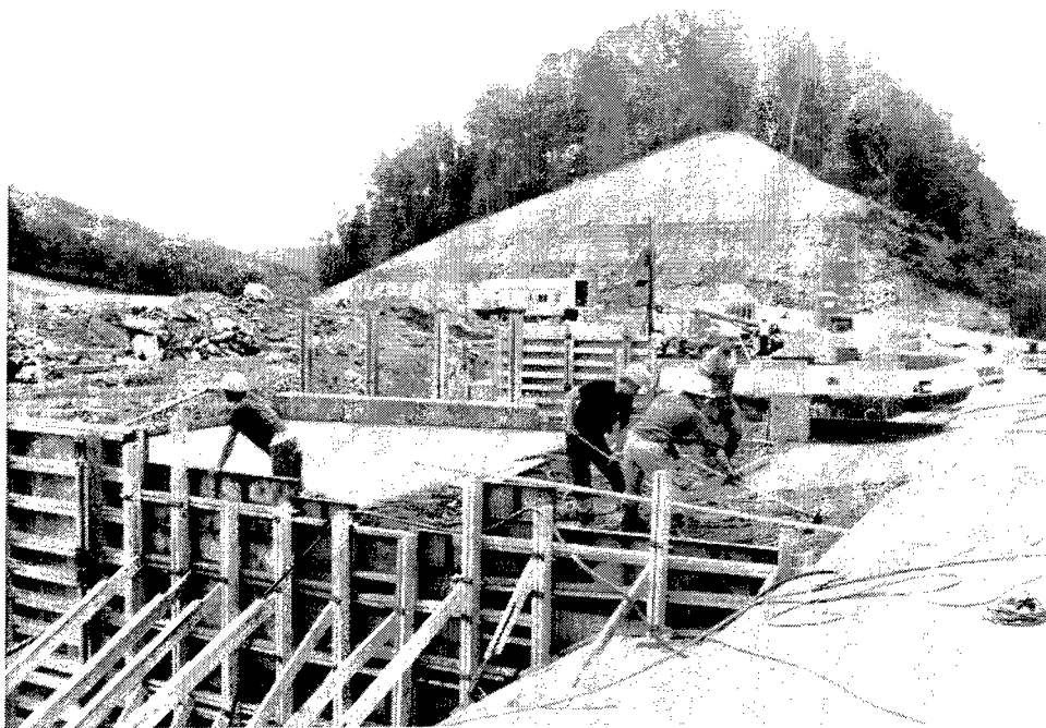
Figure 60. Placing and finishing concrete for the top of the spillway apron, Mohawk Dam (from U.S. Army Engineer District, Huntington 1990b)
