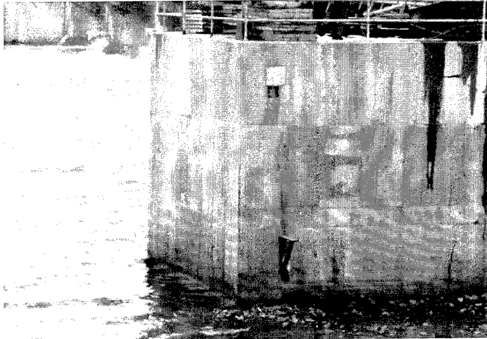
Figure 21. The south abutment of the arch dam after rehabilitation, Dresden Island Lock and Dam
