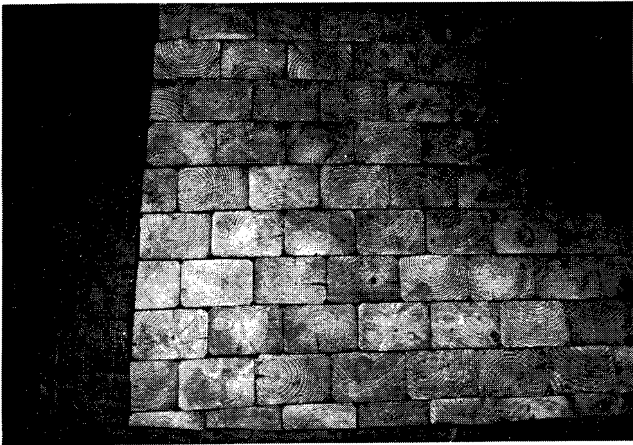
Figure 152. Building 500: A detail of the wooden floor located in the Mill Right Shop. The darker section of blocks is original, and the lighter section consists of replacement blocks.
