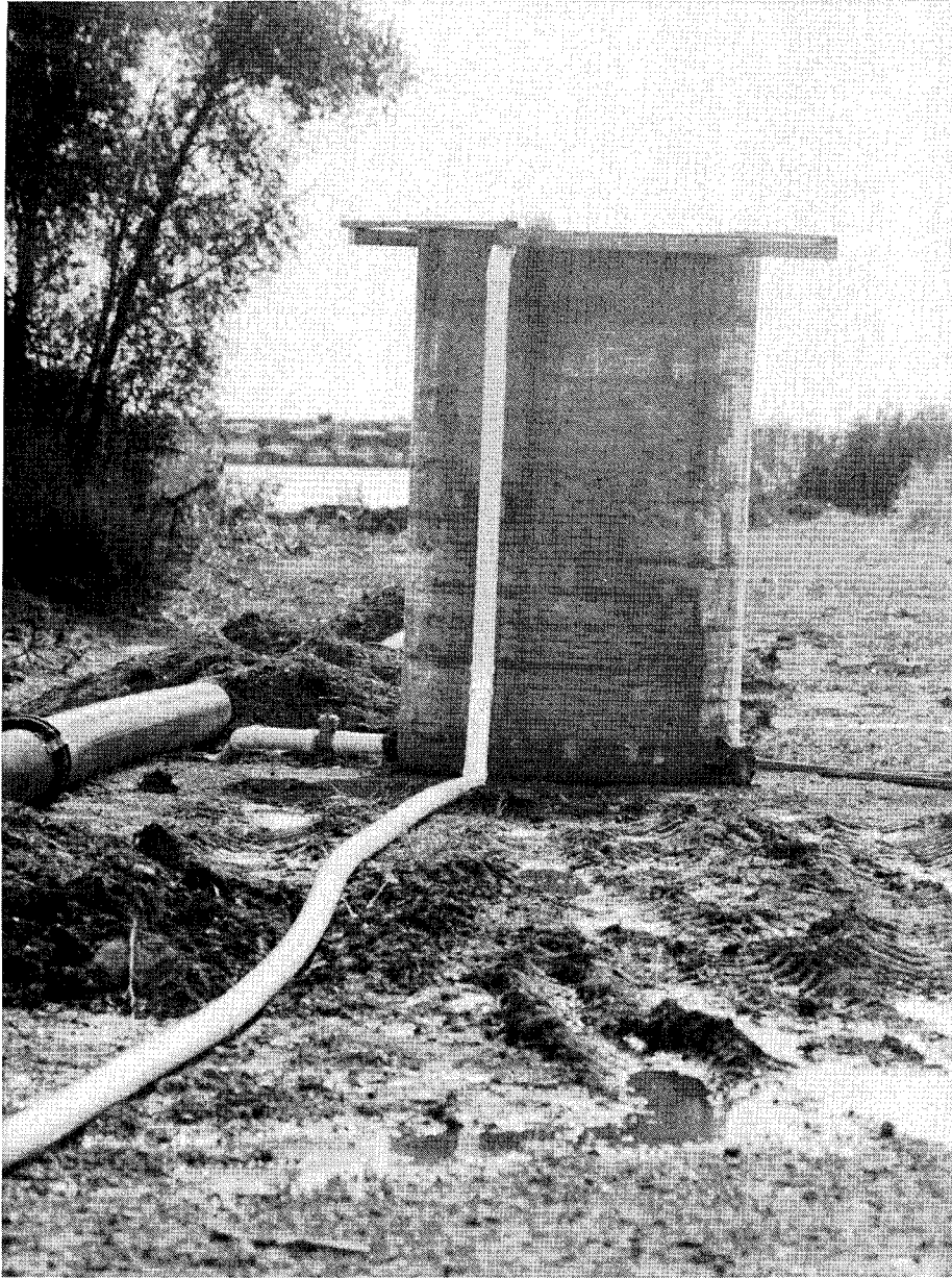
Figure M3. Clarifying tank (2,000 gal) with feed line (top) and 6 to 4 in. underflow line (bottom left)
