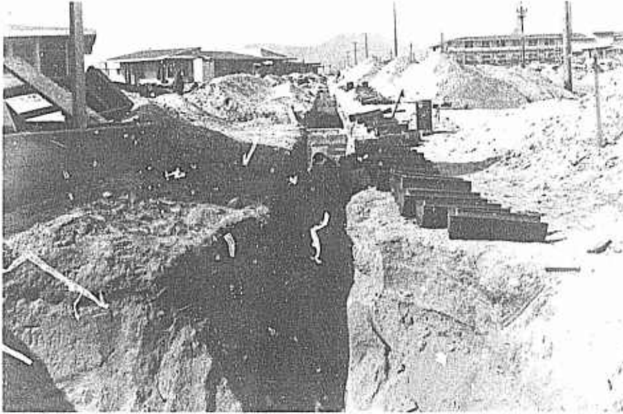
Typical construction at NOIS showing one of many inconveniences the open trench!
