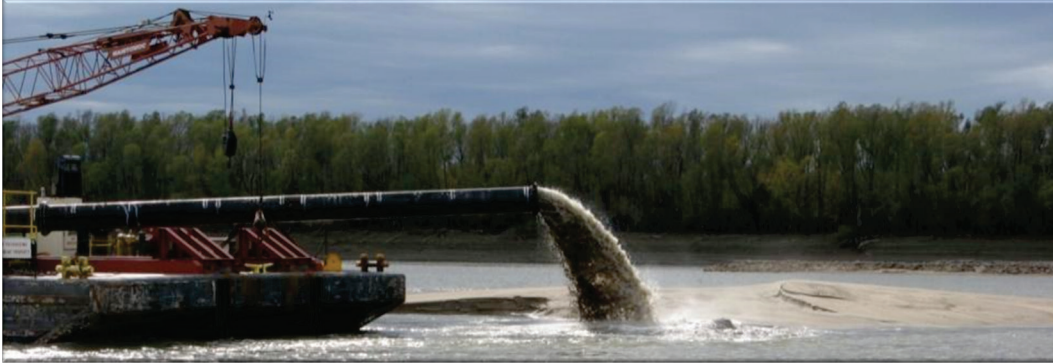
Figure 2. Island construction November 8, 2011 (river elevation ~ 105.16 m NGVD29) where approximately 76,5000 cubic meters of material was placed at River Mile (RM) 103.5 along the right descending bank. (USACE picture from 2011)
