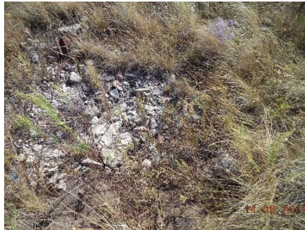
Figure 66. A. Instrument borehole. B. Broken concrete block. C. Remains of concrete slab for tower emplacement.
