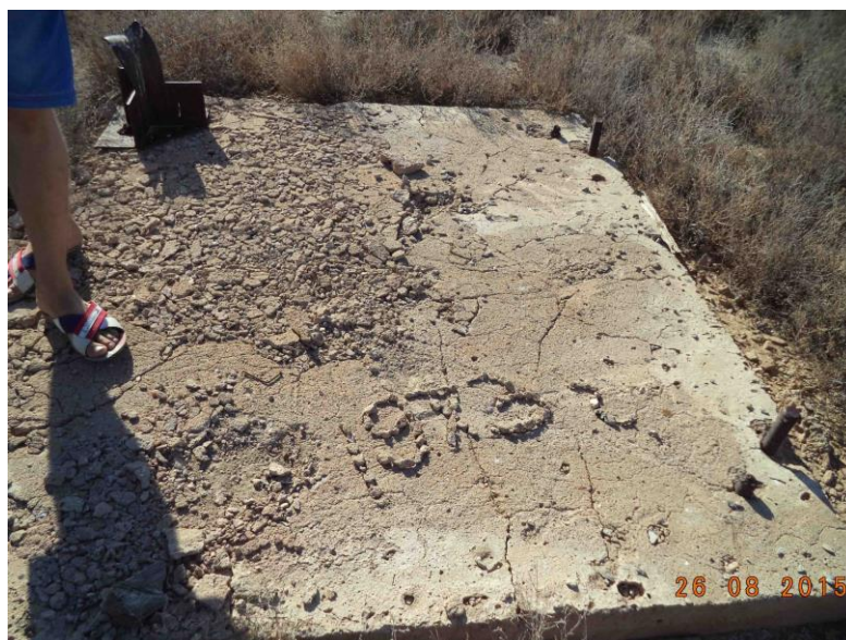
Figure 80. Concrete pad at the Meridian-2 site. The year of the explosion is written into the concrete, which is highlighted with small stones for clarity. Additional writing on the pad is no longer visible due to deterioration of the concrete.
