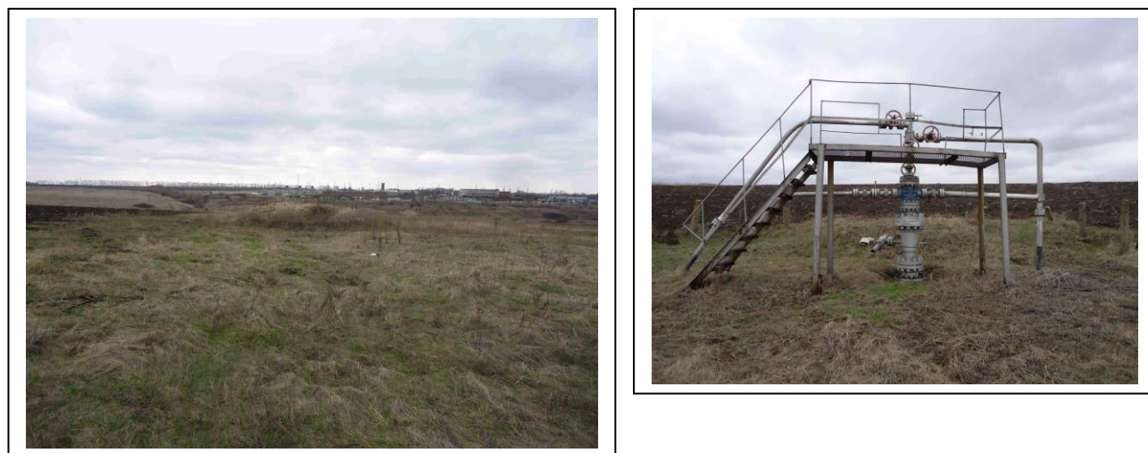
Figure 44. Left – Site of the PNE Fakel looking south. The compressor station is located in the background. Right – Gas well #258 used as a reference in locating Fakel. The PNE was approximately 100 m to the left (north) from this location. Photos by K. Mackey.
