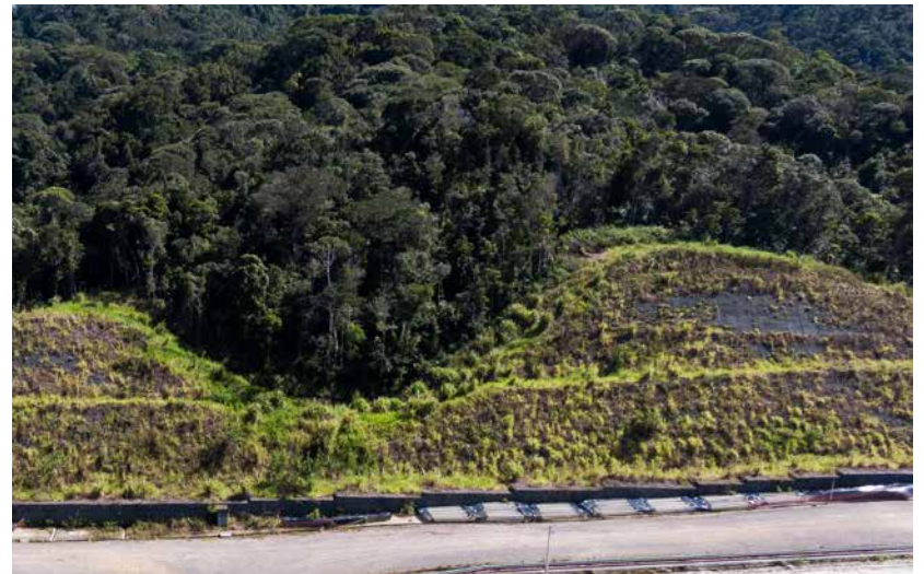
Top: Gabion walls and geosynthetic mesh for vegetative reinforcement during construction. (Photo by Dow)
