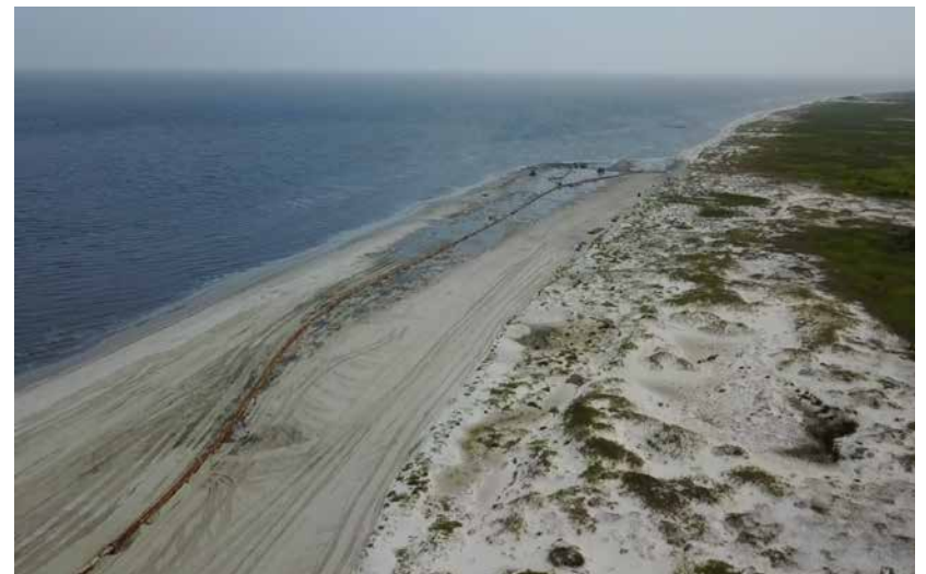
Top: Construction pad at the center of the Camille Cut at Ship Island during construction. (Photo by USACE Mobile District)
