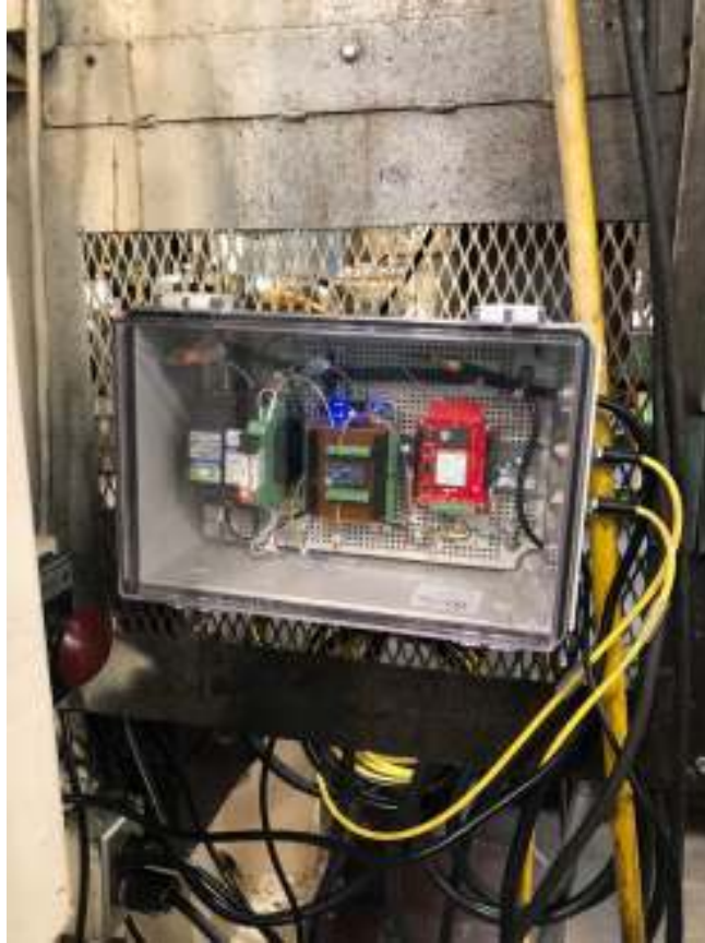
Figure 1. A project IoT retrofit kit monitoring a 400 ton press at Steelcase.
