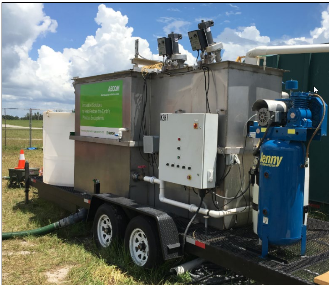
Figure 2-10. AECOM dissolved air flotation treatment system set up on shore near the Moore Haven spillway.
