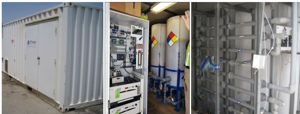
Figure 2-11. Containerized ozone advanced oxidation system from HiPOx, Inc. The system is capable of treating with ozone or ozone plus hydrogen peroxide.
