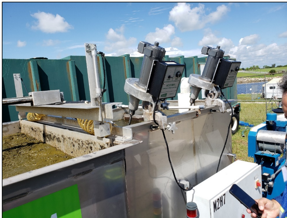
Figure A-13. Conditioning compartment of the HABITATS where coagulants and flocculants are added and mixed into the algae contaminated solution.
