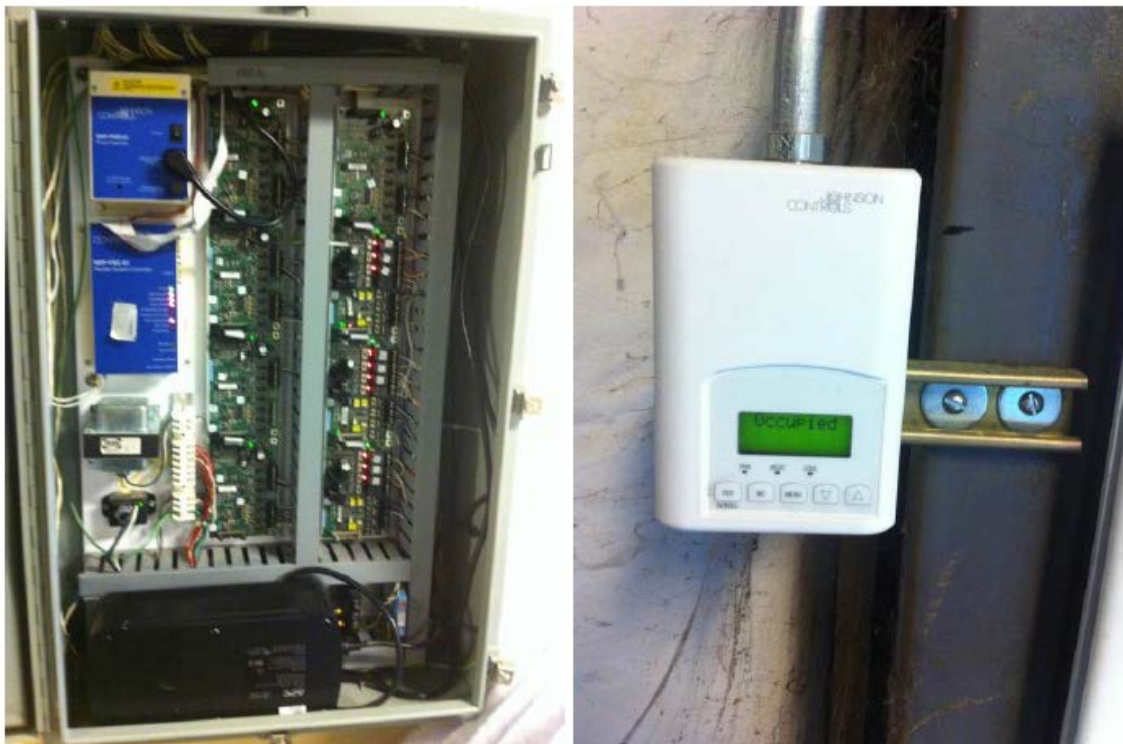
Figure 4-2. Bldg. 59; Left: Metasys N2 Controller, Right: Johnson Controls Occupancy Mode Controller
