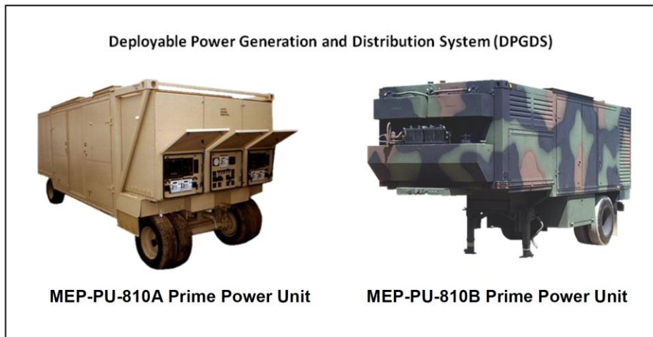
Figure 6-1 – The MEP-PU-810 generator, rated for 840 kW output, consumes 60 gallons (180 kg) of JP-8 per hour [75]
