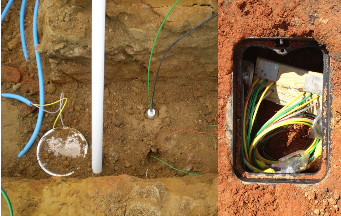
Figure B-1. Monitoring Instrumentation and Sampling Access Point
