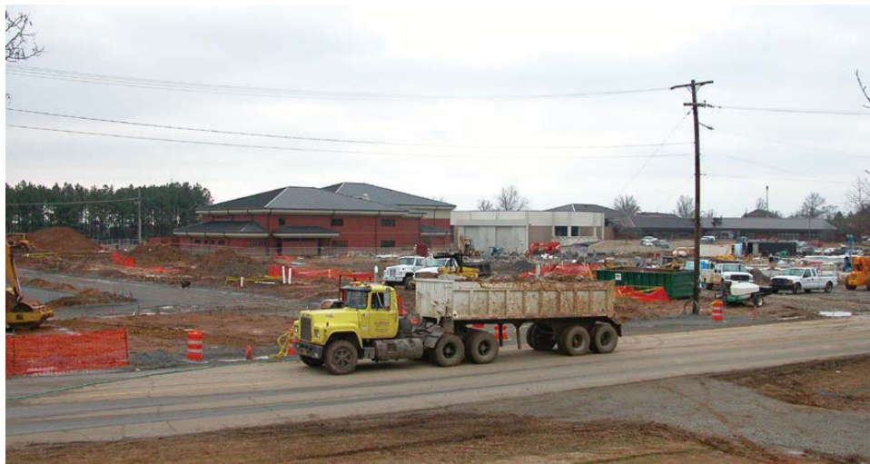
Construction commenced on the C-130J Maintenance Training Facility, with the C-130E schoolhouse and the new C-130J simulator facility in the background in December 2003. (Photo taken by 314 AW/PA; USAF Photo). 102
