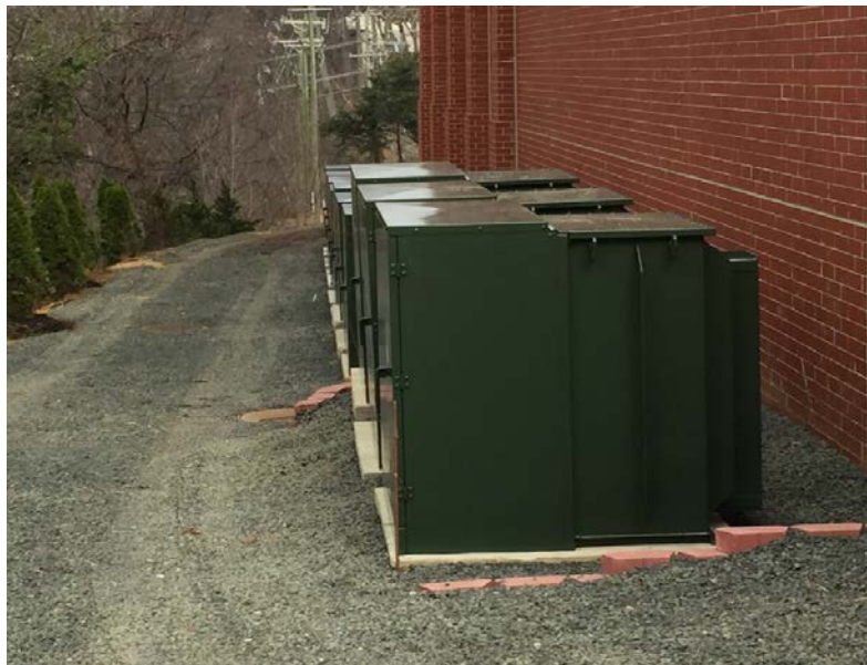
Figure 16. Ground Level Picture of Voltage Regulator Outside Radnor Heights Substation
