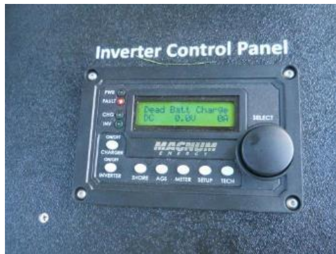
Figure 23: Smart PPS LCD Control Panel
