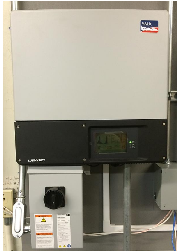
Figure 7. Solar Sunny Boy Inverter
