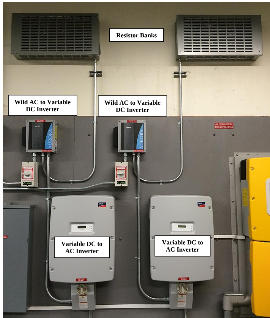
Figure 8. Wind Turbine Inverters
