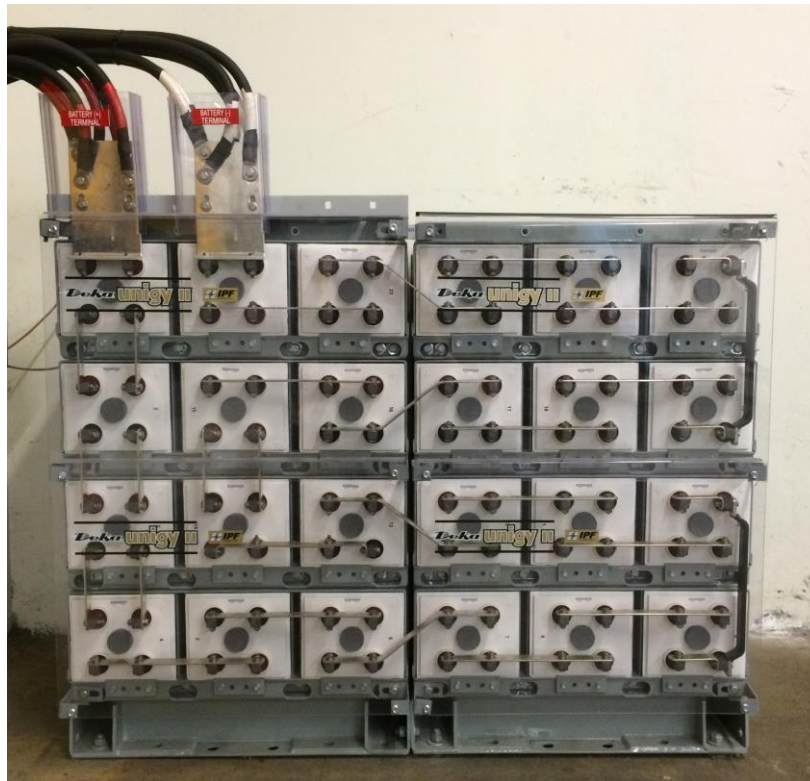
Figure 11. VRLA Battery Bank
