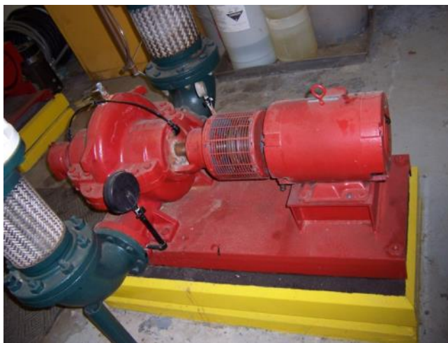
Figure B-3. Typical pump motor.
