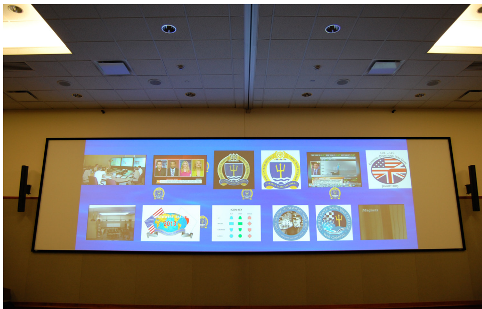
Media wall in the Joint Command Center/adjudication cell is capable of displaying multiple images to support adjudicator cell and control cell game situational awareness.
