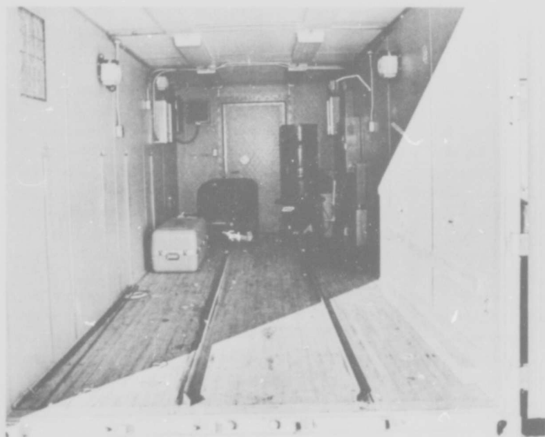
Figure 29. Interior view of camp utilities module with the generators and stove tanks removed showing the intake vent and filter on the wall in the left foreground and the mounting rails for the generators on the floor.
