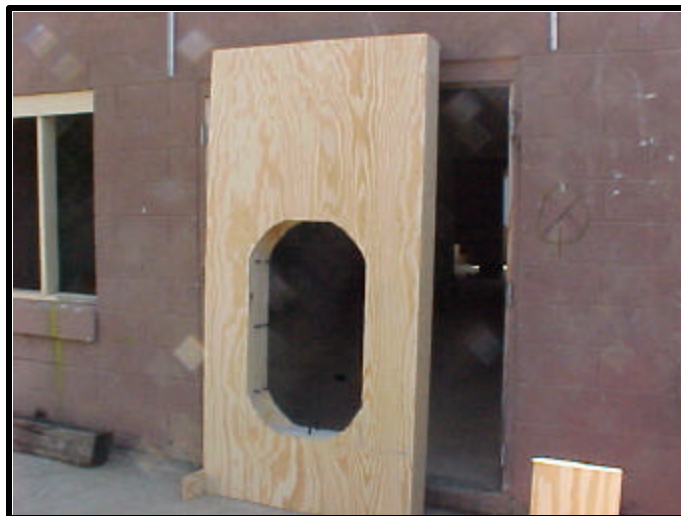
Figure 4. Hole C: 26- by 44-inch hole with 8- to 9-inch radius corners.
