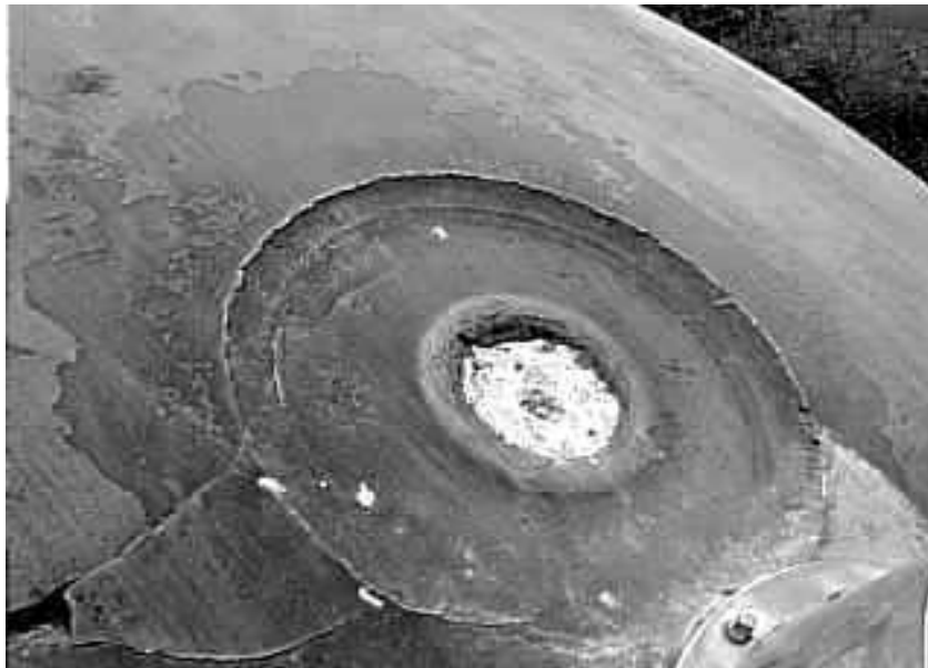
Figure 6. Photograph of Cupola 120
